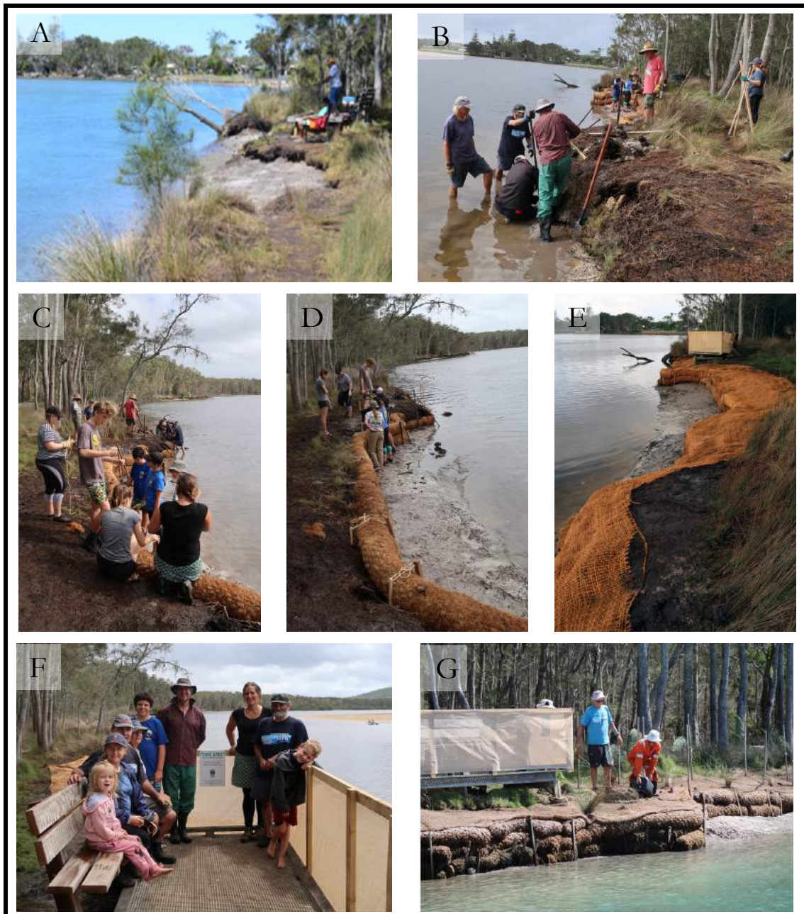
Figure 14: Remediation works carried out along Corindi River: A) Example of erosion in 2015; B- D) SURG members and local residents installing coir logs and matting along eroded section of Corindi River; E) Installation of Coir matting to stabilise river bank; F) Site barrier and information panel installed to inform visitors of remediation works; and G) Planting and watering of seedlings and grasses along remediated site.(Photos: SURG members)
